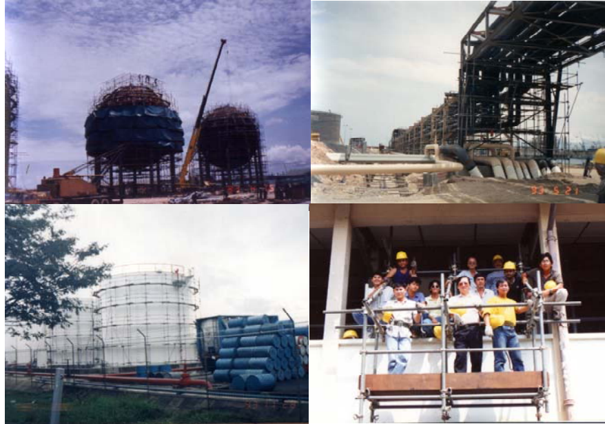
Figure 6. Some projects carried out with a scaffolding design system developed in a turnkey project (Courtesy to Hei Leck Engineering Pte Ltd)
