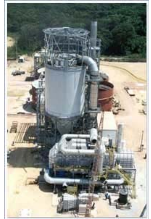
Kaolin Plant Evaporates 16,000 kg / h
