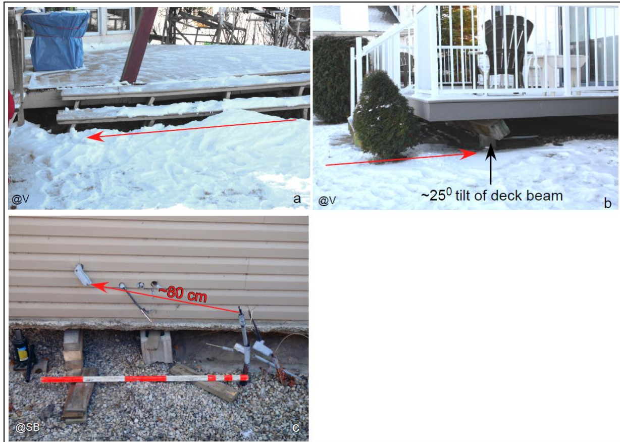
Figure S3. More damage to infrastructure. (a & b) Sheared deck structure, Lac Ste. Anne. (c) Sheared lower building structure, Seba Beach area, Wabamun Lake. Note severed electrical conduit and electrical wiring. In all panels, arrows indicate directions of ground displacements. Locations of pictures are annotated in panels based on acronyms in Figure 1.
