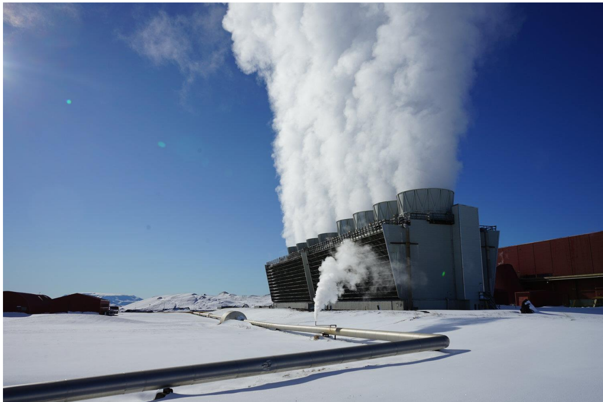
Figure A.21. Cooling towers at the Krafla Power Plant
