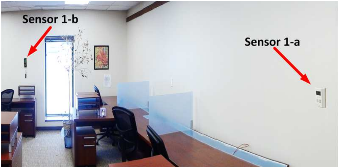
Figure 2.1: Location of the temperature sensors in the test-bed. The sensor 1-a is the room temperature sensor and the sensor 1-b is a temperature data logger installed to calculate measurement errors.
