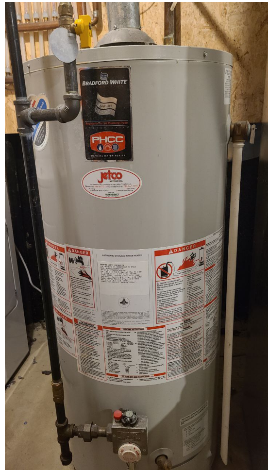
(b) Water heater
